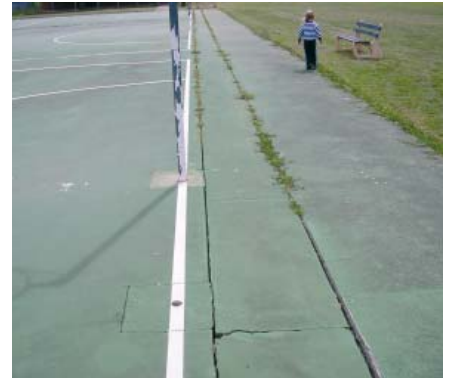
Photo 1 - Example of trip hazards on Netball Courts
