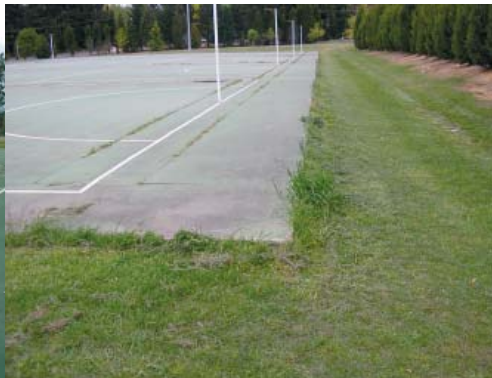
Photo 3 - Trip hazards on Netball court
